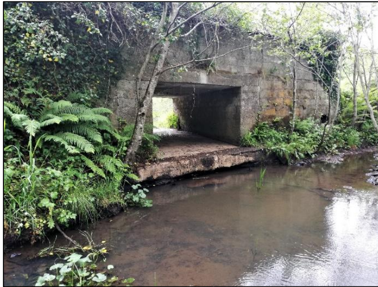
Plate 9B-9: Mullaghagarry at W1-17, Existing Impassable Culvert on Local Road
