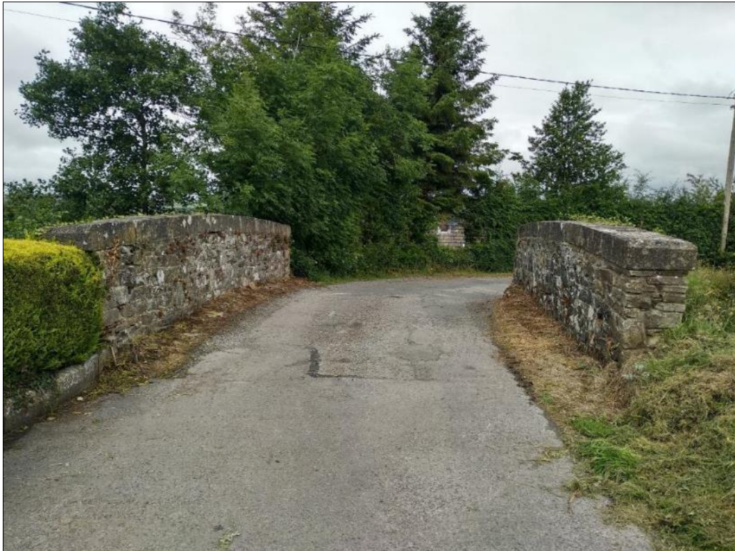
Plate S2-18: View of deck and parapets of road over rail bridge NIAH 40905394
