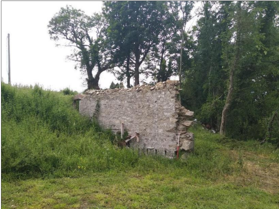
Plate S2-36: View of external wall elevation of former mill structure (NIAH 40905390)
