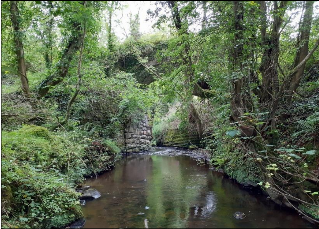
Plate S3-15: View to northwest of disused railway bridge (NIAH 40905447) northeast of possible mill race (L307-4), Ch. 2+300
