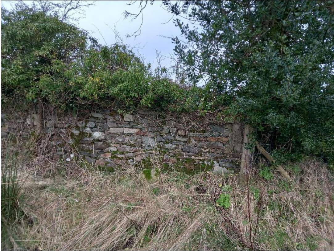
Plate S3-106: View to south of demesne walling (Croaghan House) forming townland boundary Townparks/Carricknaslate at Ch. 16+650
