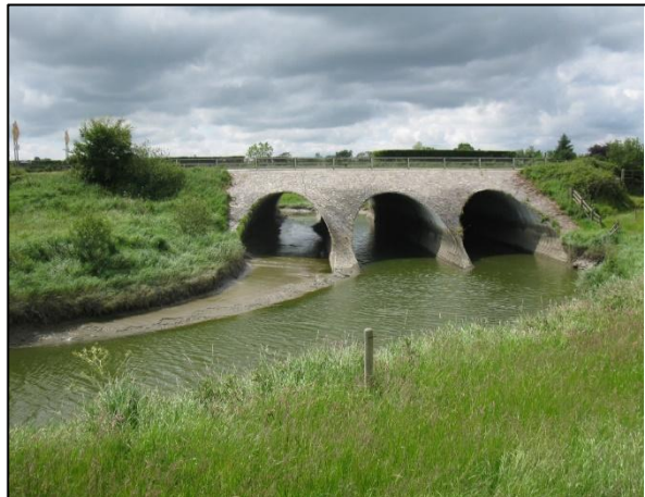
W2-15 (Sept. 2024) – Isle Burn (EPA “Leslie Hill stream”) existing crossing structure at Swilly Estuary on SAC boundary, view upstream from northern side.
