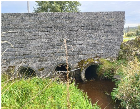
W1-01 (Sept. 2024) Tributary of Burn Daurnett, view of existing triple pipe culvert and headwall.
