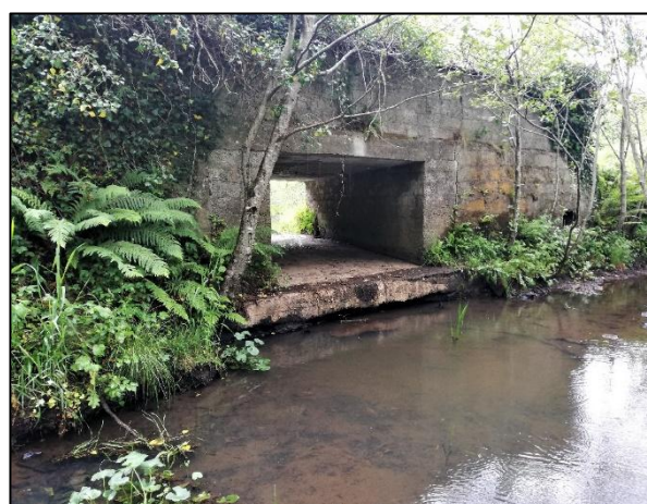
W1-17 (Sept 2024) Mullaghagarry, existing culvert on local road. Flow is undermining culvert bed. Fish passage barrier.
