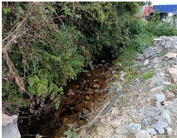
W2-05 (Sept. 2024) Channel had been recently culverted (pipe) for industrial entrance in 2024.
