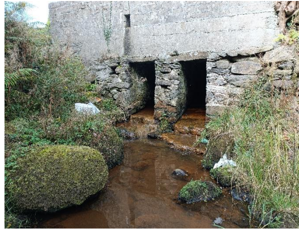
W1-05 (Sept. 2024) Cappry, downstream of crossing point – sewage fungus on culvert apron
