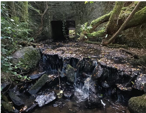
W2-10 (Sept. 2024) Farsetmore at existing local road crossing. Fish passage barrier.
