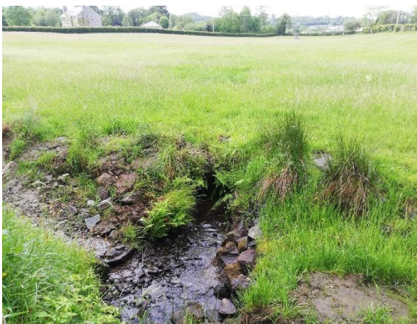
W1-07 (June 2020) Dromboe Lower, view over piped section in field. This will be daylighted as part of proposed works.
