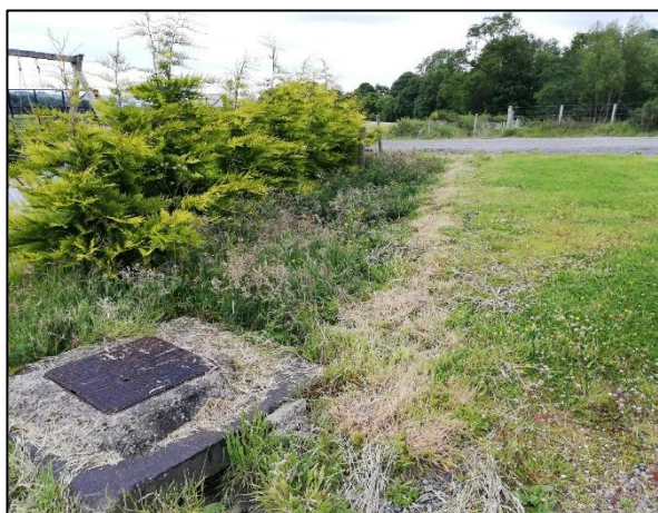
W2-08 (Sept. 2024) piped at upper end of watercourse in crossing reach.
